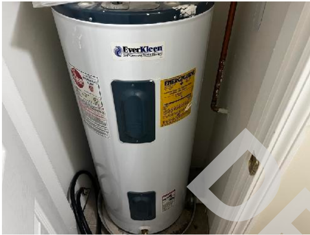
Domestic water heater
