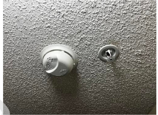
Sprinkler head and smoke detector
