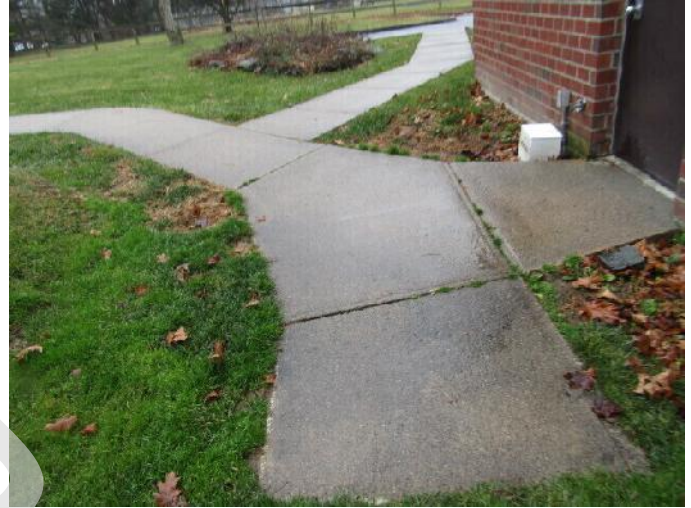
Vertical displacement at Building D
