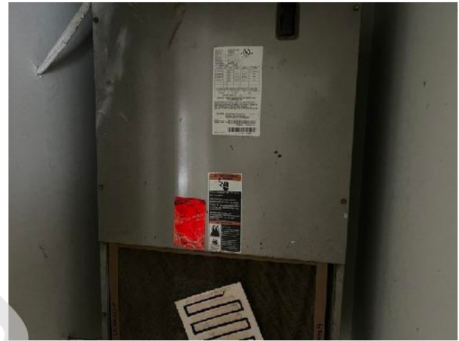
HVAC furnace unit
