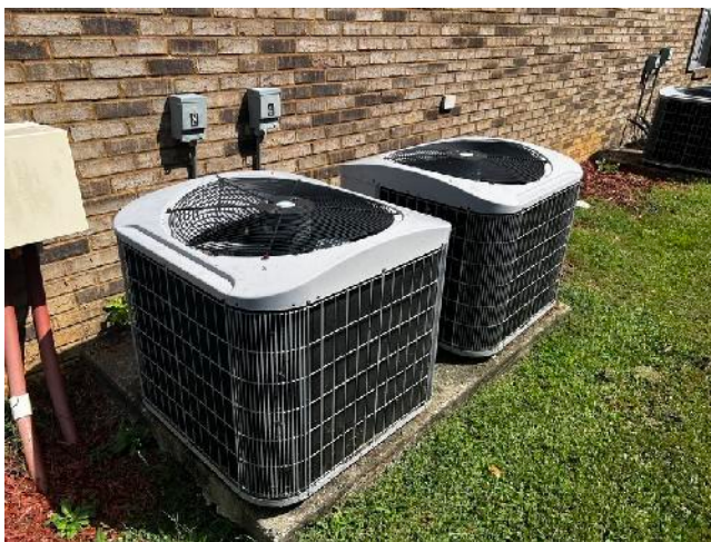
HVAC condensing units
