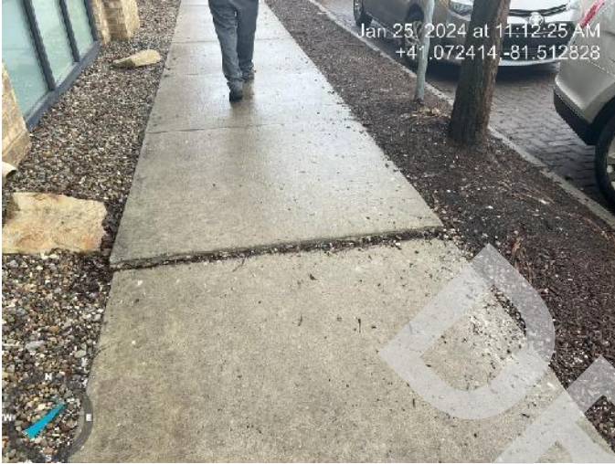
Vertical displacement at Building A
