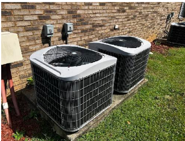
HVAC condensing units
