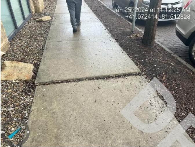
Vertical displacement at Building A
