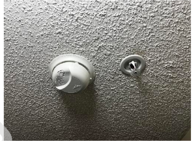
Sprinkler head and smoke detector
