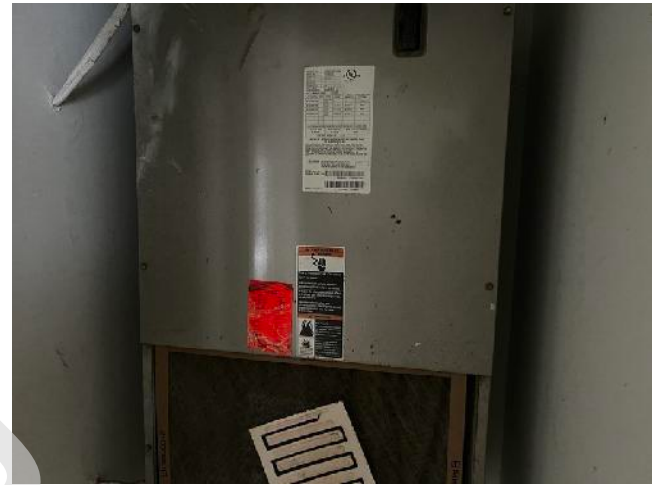
HVAC furnace unit
