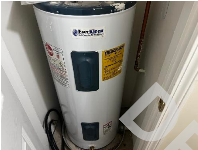
Domestic water heater
