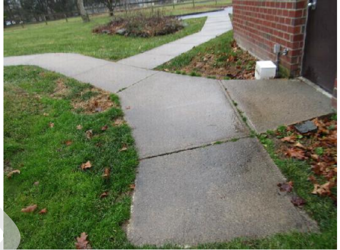
Vertical displacement at Building D
